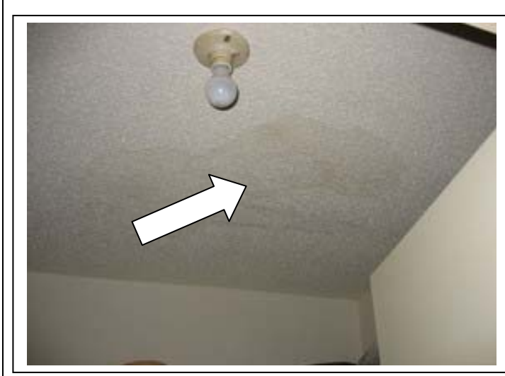
Photo # 11 Stain in bedroom closet ceiling.
