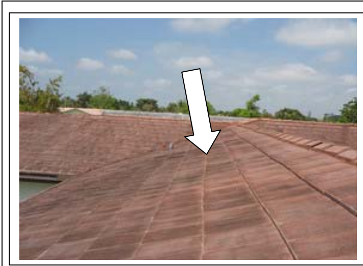
Photo # 4 The roof is also sagging over the living room. This field faces south.
