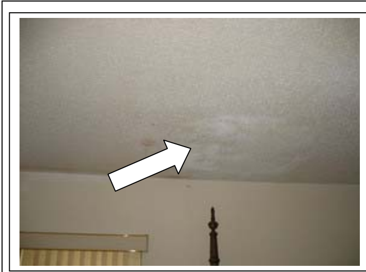
Photo # 10 Stain in bedroom ceiling.
