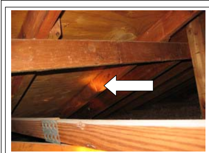
Photo # 5 Top chord of truss over the kitchen area is cut and spliced.
