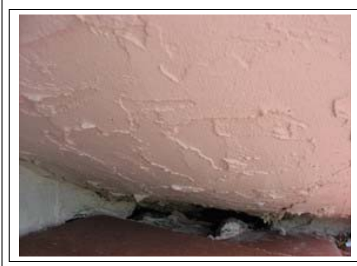
Photo # 12 Possible entry point under eaves for water to damage ceiling in bedroom area.
